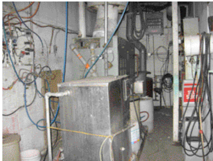
Before: The equipment room was in need of a complete overhaul.
