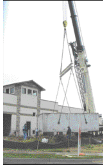
The installation of a 10,000 gallon water storage tank saved more than $100,000 in water tap fees on this project.
